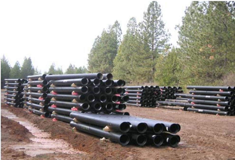
Water pipes waiting for the start of the Cement Hill NID water project.
